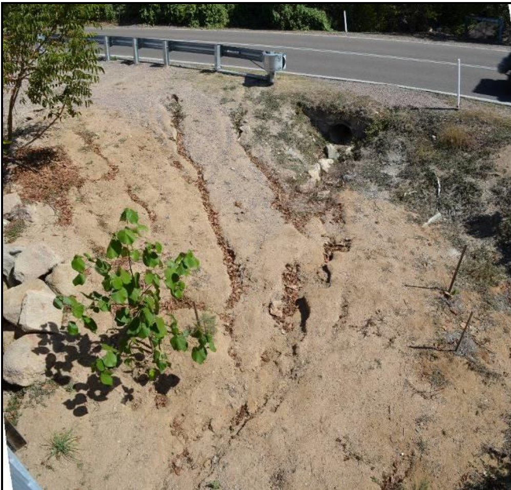
Figure 3-6 Gabul Way Erosion
