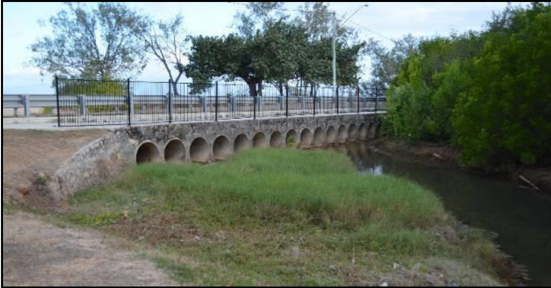
Figure 3-3 Petersen Creek Drainage Obstruction
